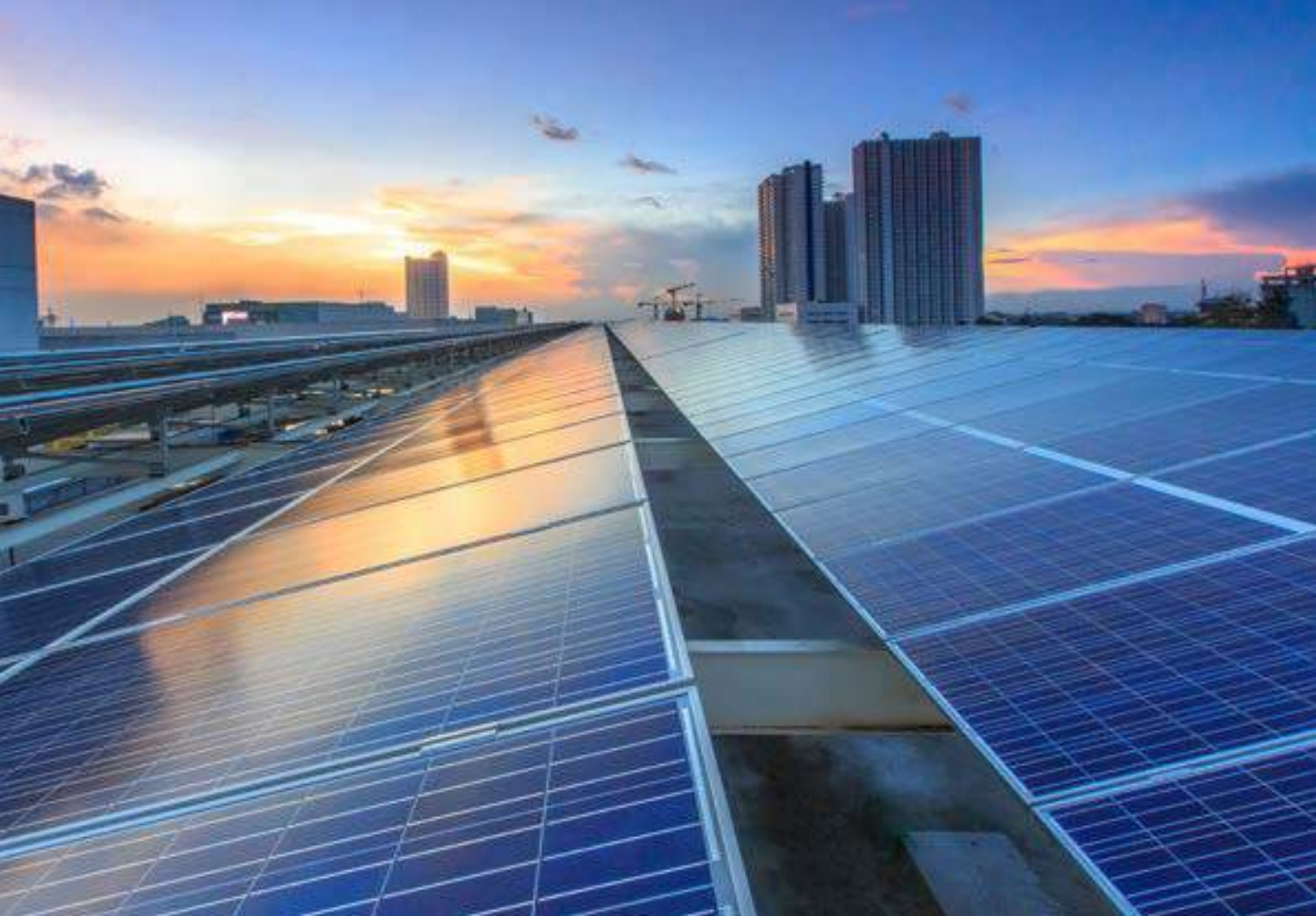
Solar roof deck at the Mall of Asia
